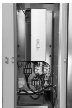
Figure 4. Variable Frequency Drive
