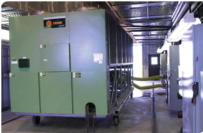
On-site test facility ensures reliability and performance verification
